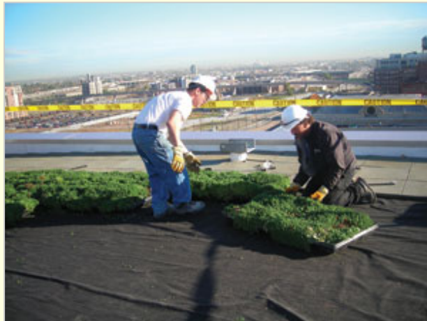
Installing a modular Green roof system atop the EPA building in Denver, Co.
