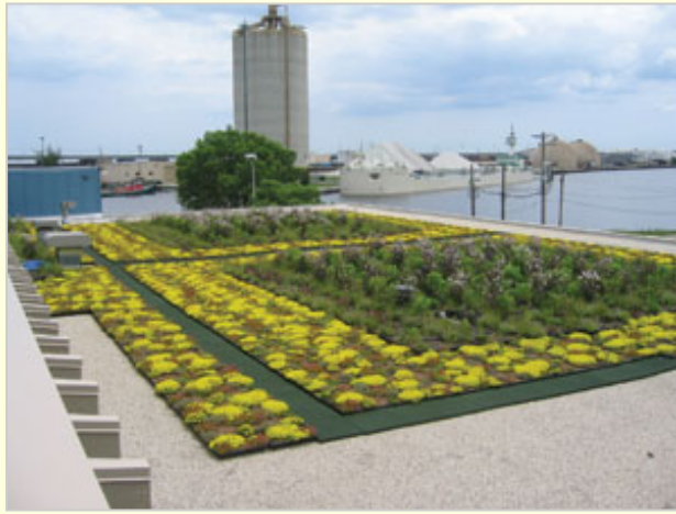
A Green roof system atop a campus building at the University of Wisconsin.
