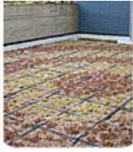
GreenGrid's modular system makes green roofs an option for residential buildings, such as this condominium complex.
